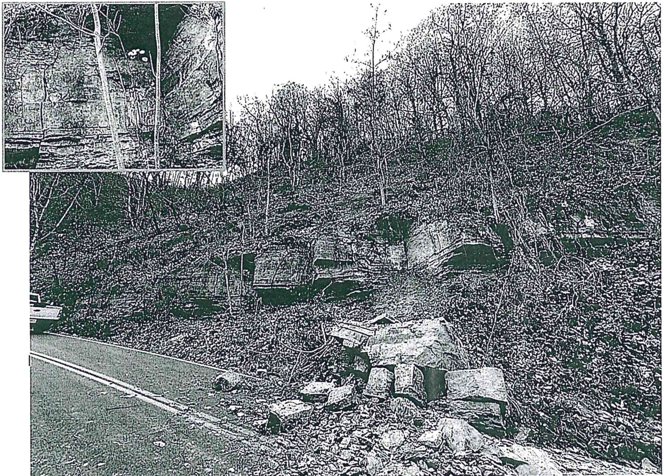
Photo 3: Fallen Rock in the Road While Showing Additional Discontinuities in the Upper Rock Mass
